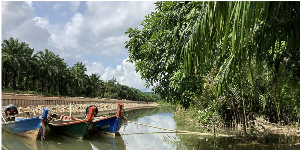
Figure 18 The use of hard structure to protect riverbank (left) and pre-construction condition (right)
